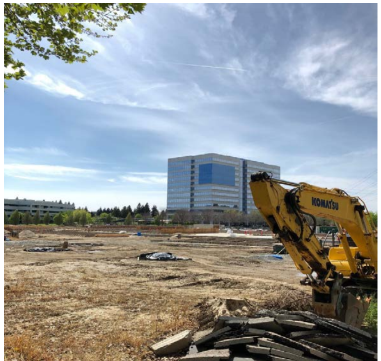
Construction has started at 2555 Natomas Park Drive in South Natomas, a 90,000 SF spec development due to complete by the end of this year.
