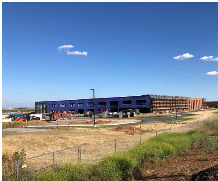
The California Military Department Headquarters building (pictured above on May 20, 2020) is under construction at 10601 Bear Hollow Drive next to Mather Airport. The 285,000 SF building on 31 acres will house the California Army National Guard, California Air National Guard, California State Military Reserve, and California Youth and Community Programs. The design-build team of Walsh Construction and Stantec will deliver the new $135 million building for the State of California by Q4 2020.
